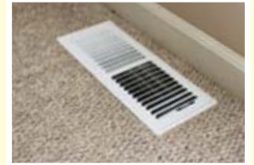
Warm air comes out of the ceiling or floor register (shown here), which takes up very little space in the room.
