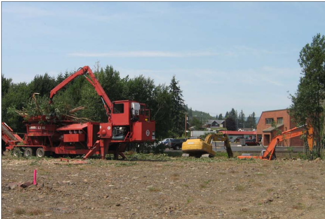
Work started Tuesday removing the remaining trees between the Wauna Federal Credit Union (in background) and the new CPUD headquarters site.
