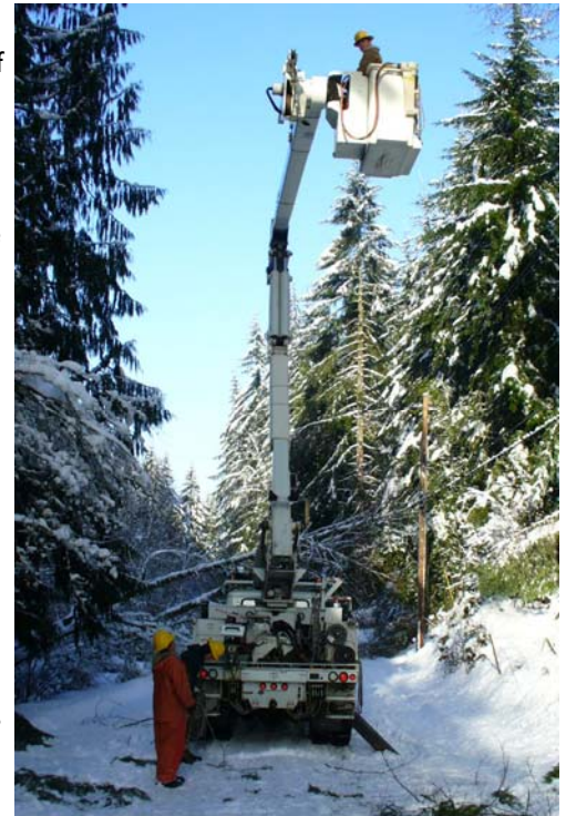
CPUD apprentice lineman Braden Lever ( in bucket) and lineman Tony Perniconi repair lines damaged from a recent winter storm.
