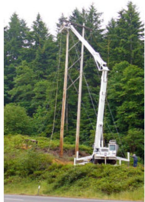
BPA working along Hwy 30 on June 30th to repair damage to the 115kV Transmission Line. Photo by Kerry Kallunki, Clatskanie PUD.
